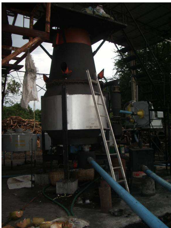
Bio digester in Kampong Cham
