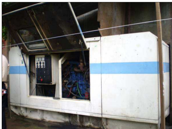
Diesel generator, Cambodia
