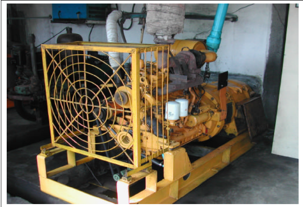
Photo 3 : Generator set REE
