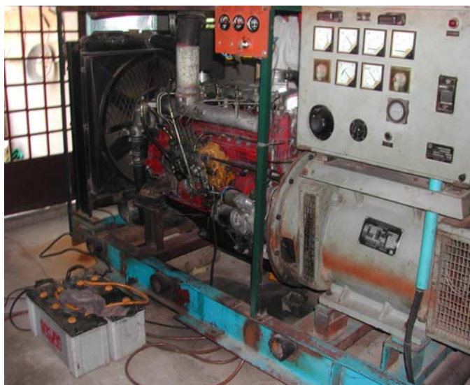
Genset operation in Cambodia October 2005
